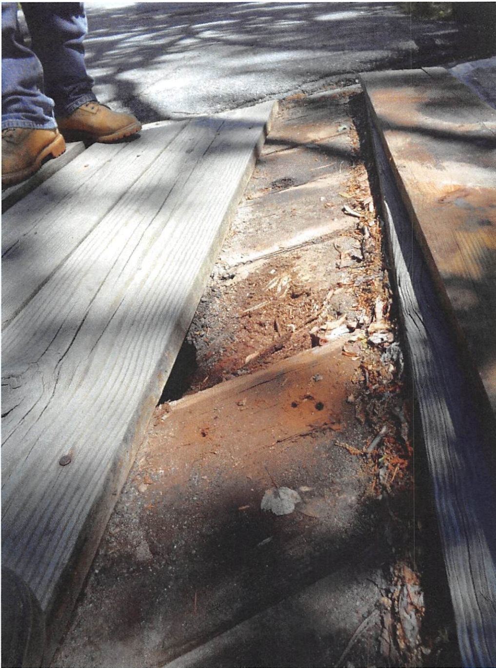
Photograph 2 - Rotting timber deck with 100% section loss.
