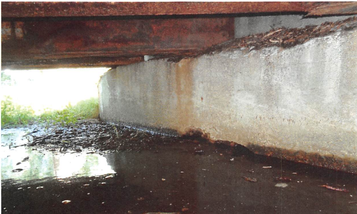
Photograph 7 - Deteriorated concrete at water line of North Abutment
