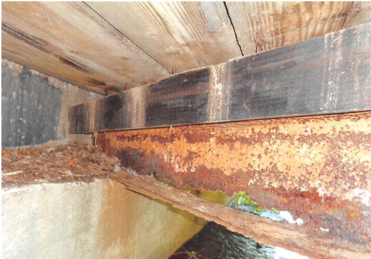
Photograph 1 – Interior girder failed due to crushing and large slotted hole in web. Note the 3" to 4" separation between the timber blocking and the timber decking. Girder located under wheel path.
