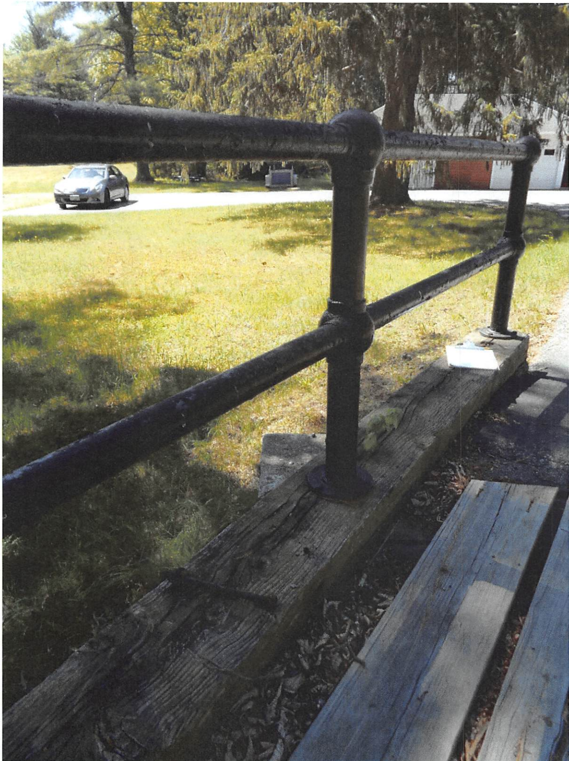
Photograph 5 - Debris collected on deck, rot in timber curb (note dislodged connection bolt)
