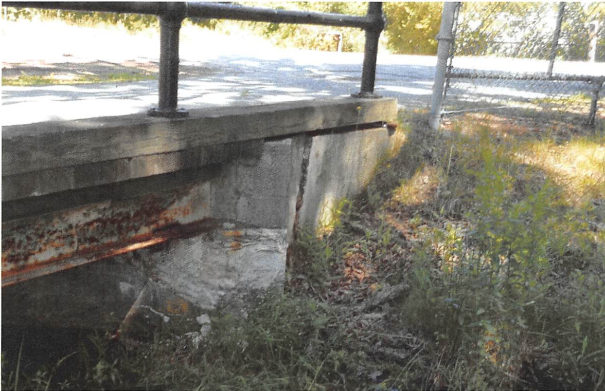
Photograph 6 - Cracked northwest wingwall, separated from abutment
